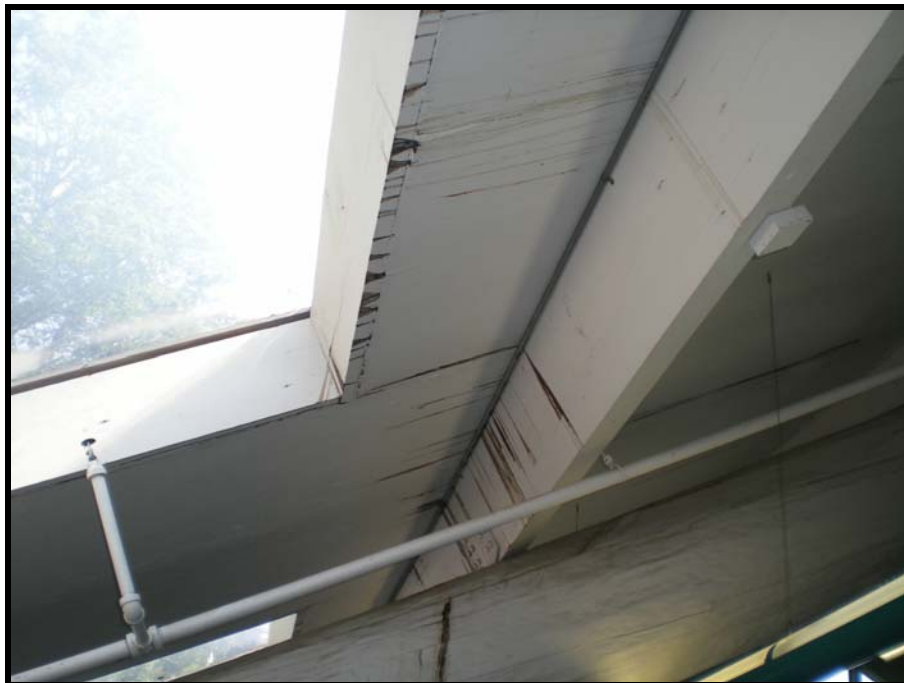
Photo- 16 Leakage Observed in Dormers on South Face of Roof
