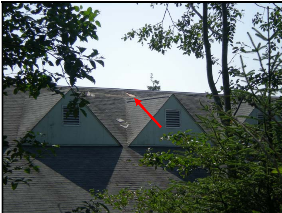
Photo- 4 Example of Area of Exposed OSB Sheathing
