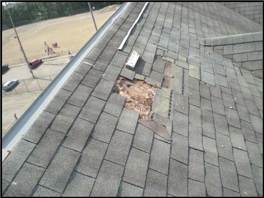
Photo- 6 Example of Bird Damage Resulting in Exposed OSB and Plywood
