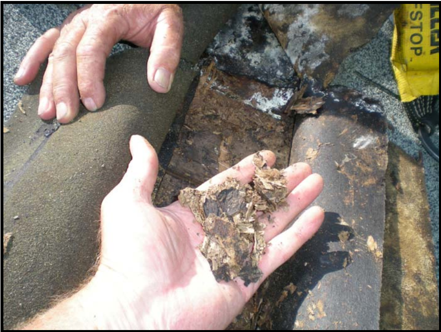
Photo- 10 Decayed and Flaking OSB Sheathing
