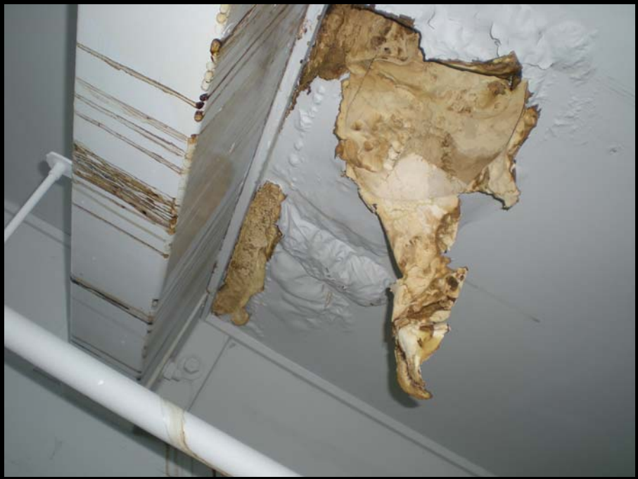
Photo- 19 Paint Blistering at the Transition Between the Addition and the Existing Building
