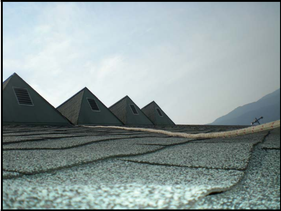
Photo- 11 Roof Deflection as a Result of Decayed and Deformed OSB Sheathing
