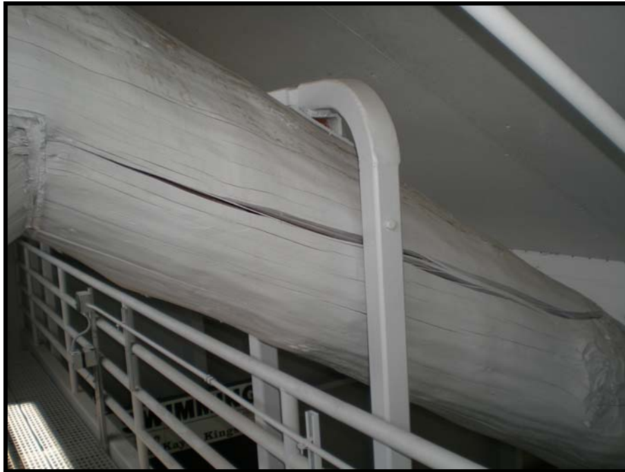
Photo- 21 Example of Cracking of the Log Beams
