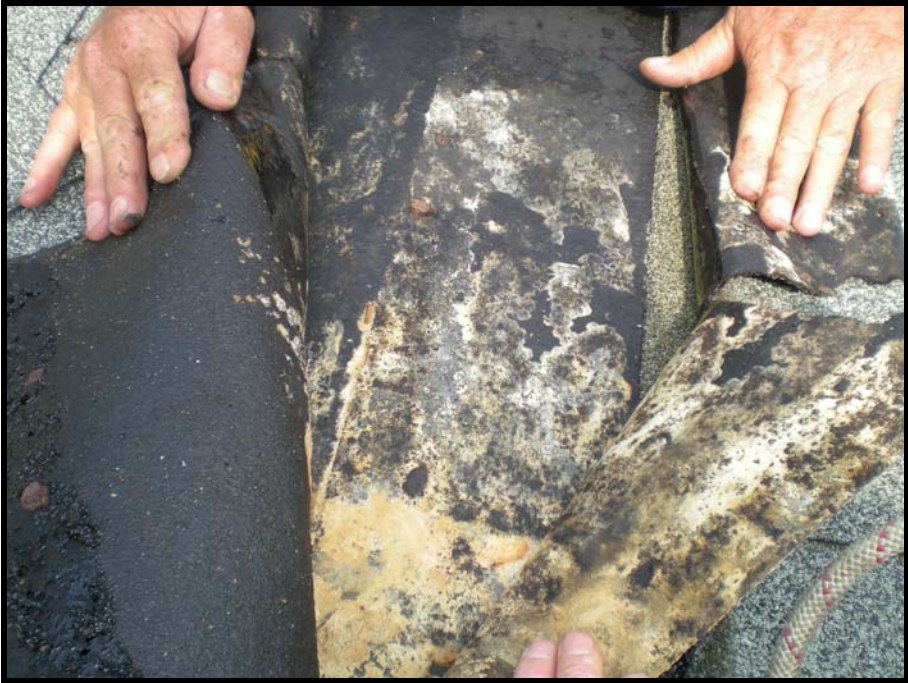
Photo- 13 Organic Growth Between Shingles and Roofing Felt
