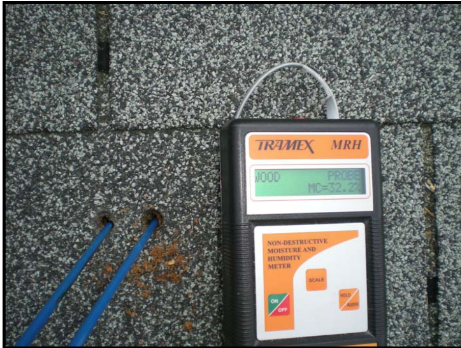
Photo- 3 TRAMEX Moisture Meter Reading of the Plywood Surface Taken at the Top Surface of a Composite Panel - 32.2%
