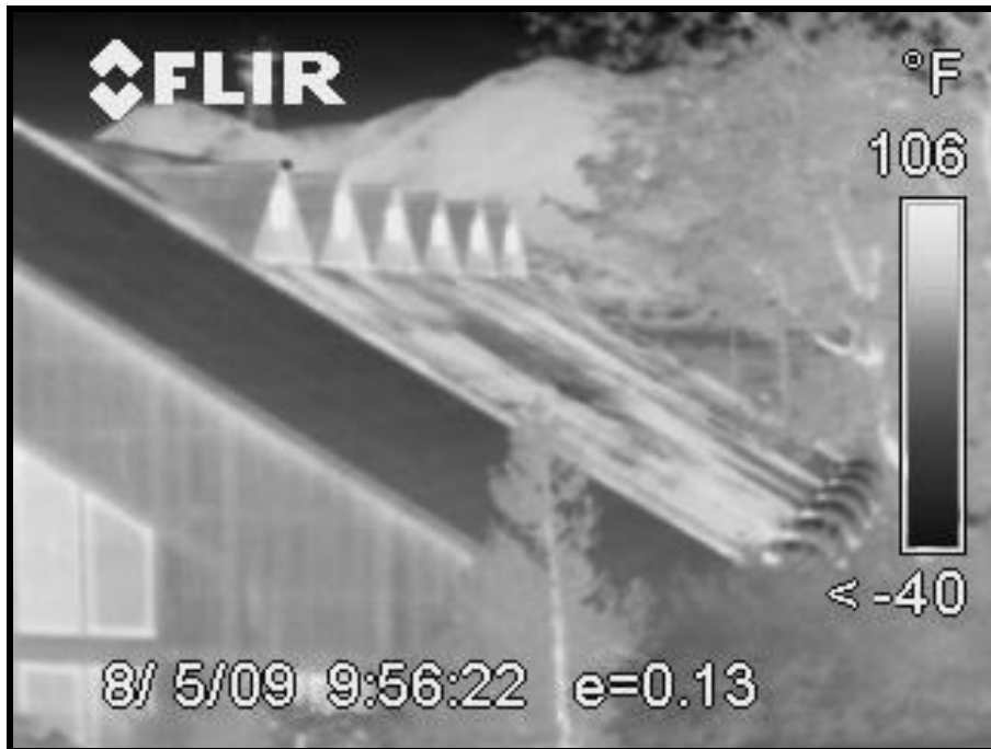
Figure 4 Infrared Overview of North Elevation – Note Addition Roof is Dry
