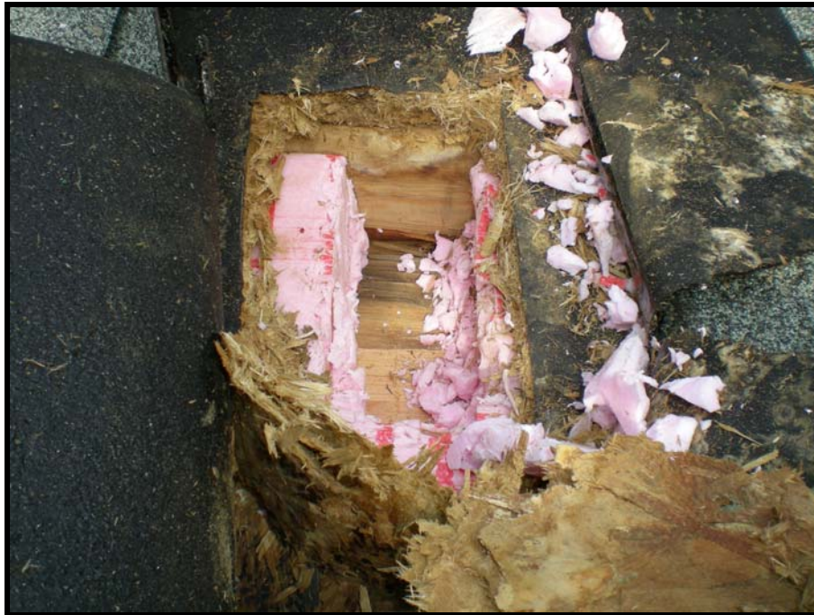
Photo- 15 Intrusive Opening in Composite Panel Revealing Wet Plywood and Extruded Polystyrene Insulation – This Area is Assumed to be a Repair Based on the Change in Insulation, the Materials Replaced do not Form a Composite
