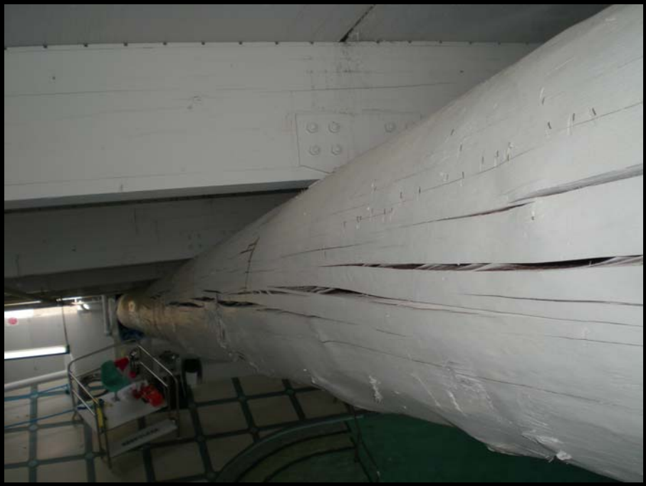
Photo- 20 Example of Cracking of the Log Beams
