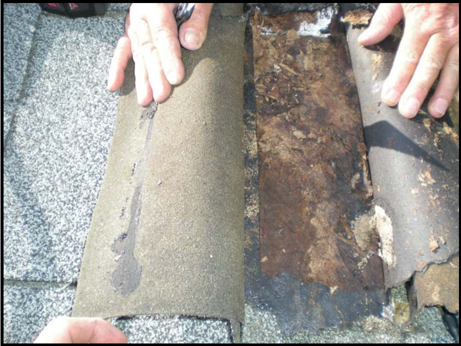
Photo- 9 Shingles Lifted to Expose Wet and Decayed OSB Sheathing
