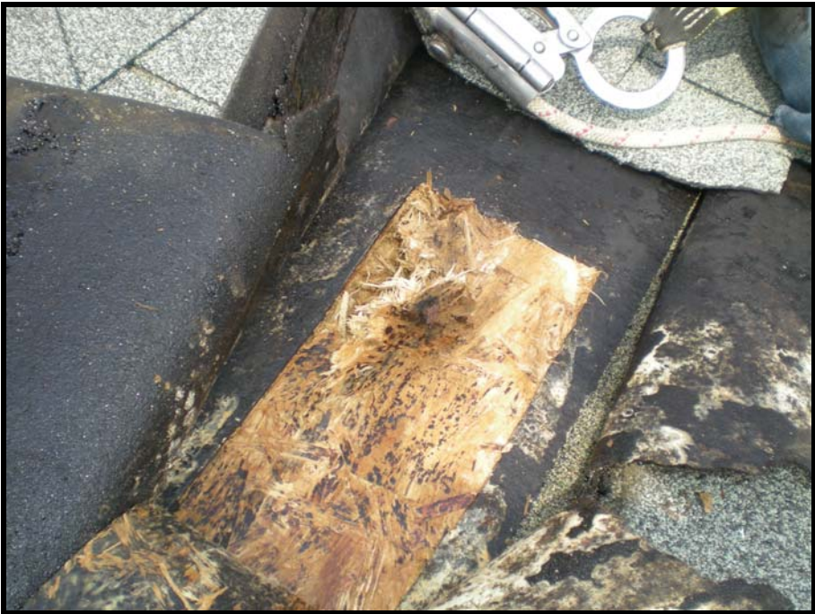
Photo- 14 Organic Growth Between Roofing Felt and OSB Sheathing
