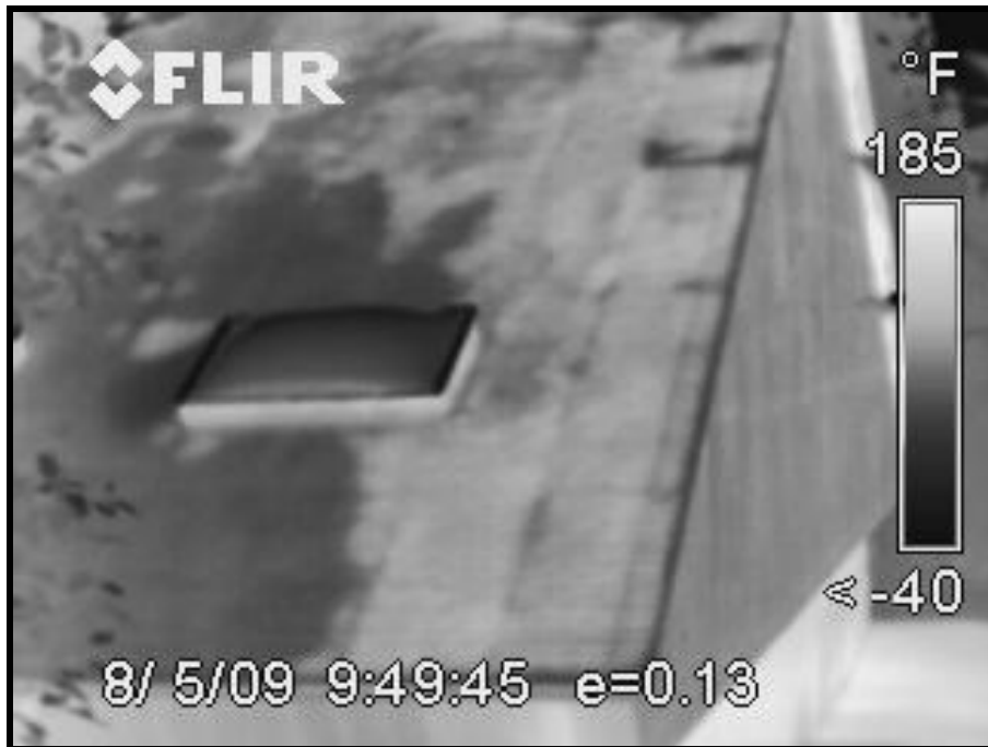
Figure 2 Infrared Photo of Northwest Corner of the Roof
