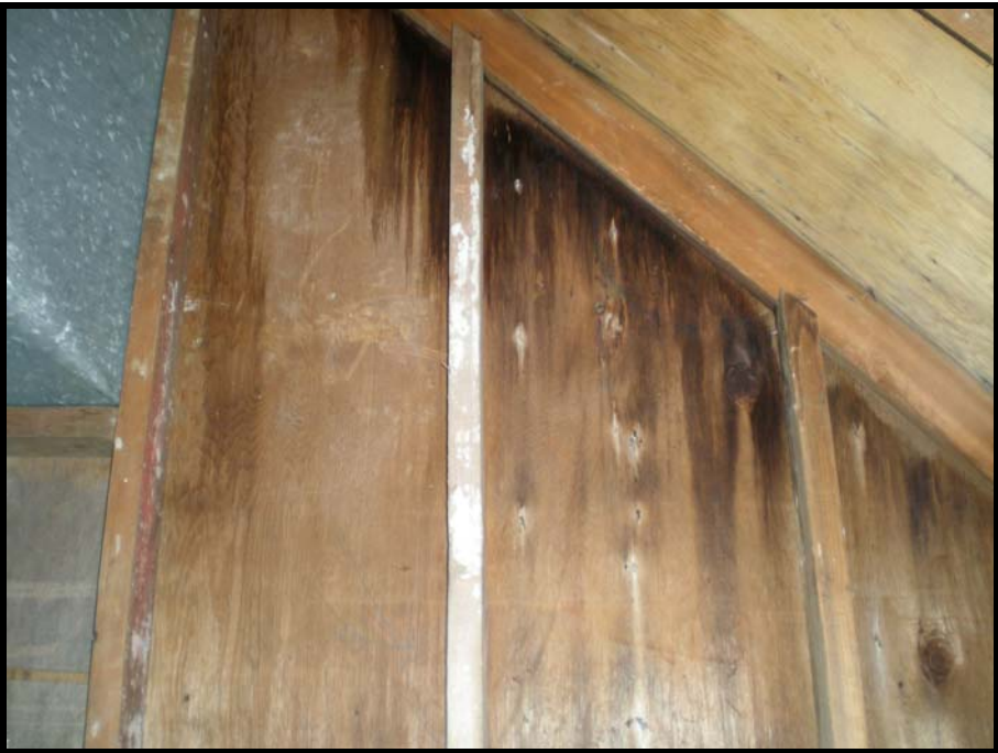
Photo- 17 Water Staining on the Interior of the Dormer Housing the Mechanical Vent
