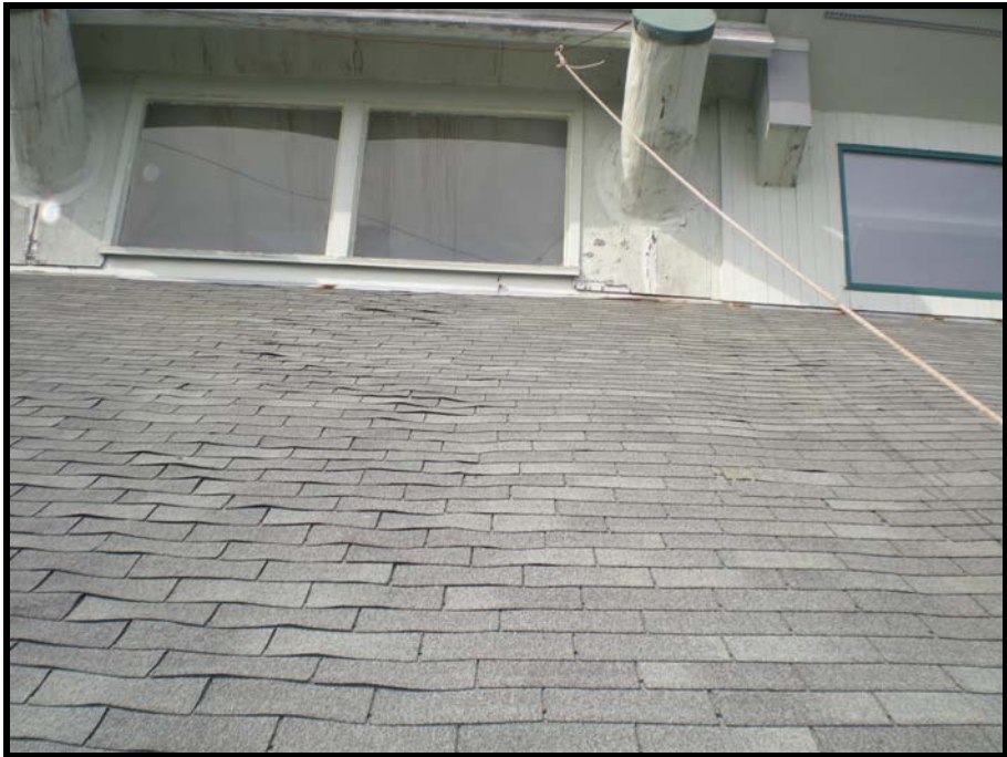
Photo- 12 Roof Deflection as a Result of Decayed and Deformed OSB Sheathing
