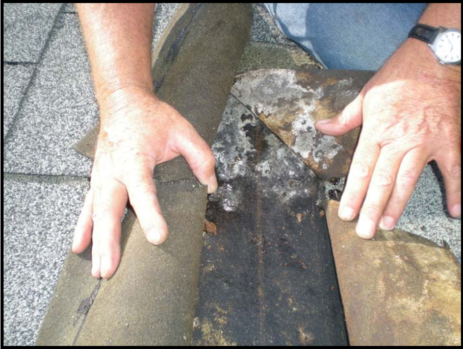
Photo- 8 Shingles Lifted Revealing Wet Roofing Felt
