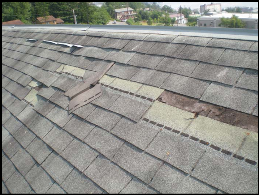
Photo- 5 Example of Missing and Damaged Shingles
