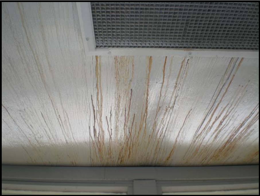
Photo- 18 Leaking and Staining at and Around an Interior Vent
