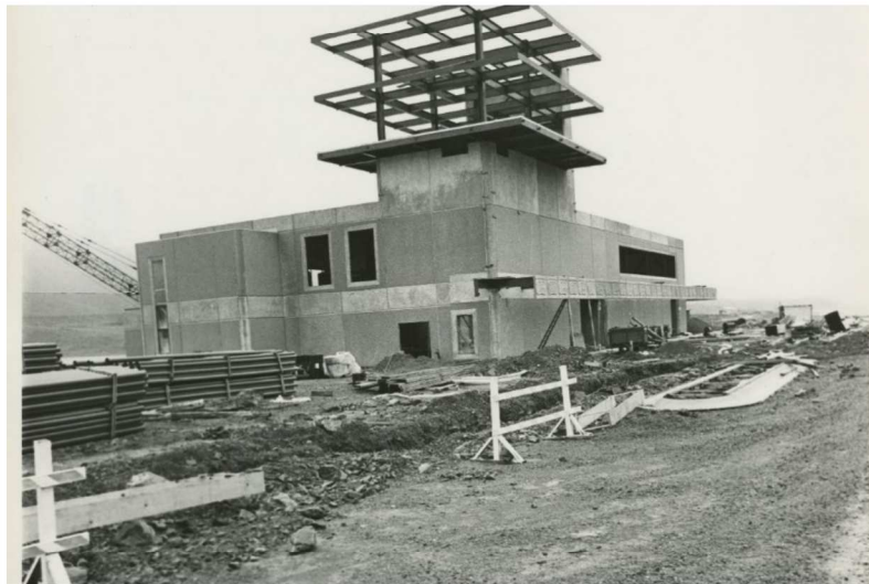
Figure 21. KTN Terminal under construction, 1972-1973. Note the Tsimshian totem design has been applied to the cantilevered awning.
