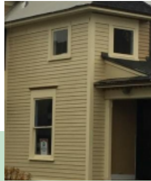
The restoration of the Yates Memorial Hospital (1905) is employing a combination of repair of existing windows and replication of damaged windows with all wood replacements (built locally). Storm windows and interior insulating shades will be used to meet energy efficiency standards.
