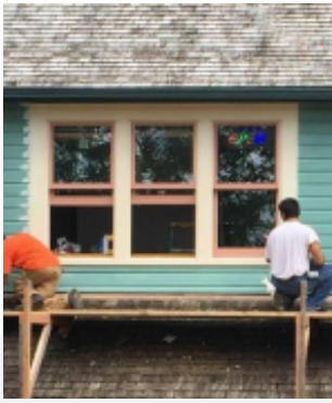
In 2015, all wood Marvin double-hung windows were chosen to replace inappropriate picture windows on the historic #4 Creek Street building (c.1920). The replacement windows are energy conserving, designed to match the proportion of the earlier double-hung windows and the original exterior trim
