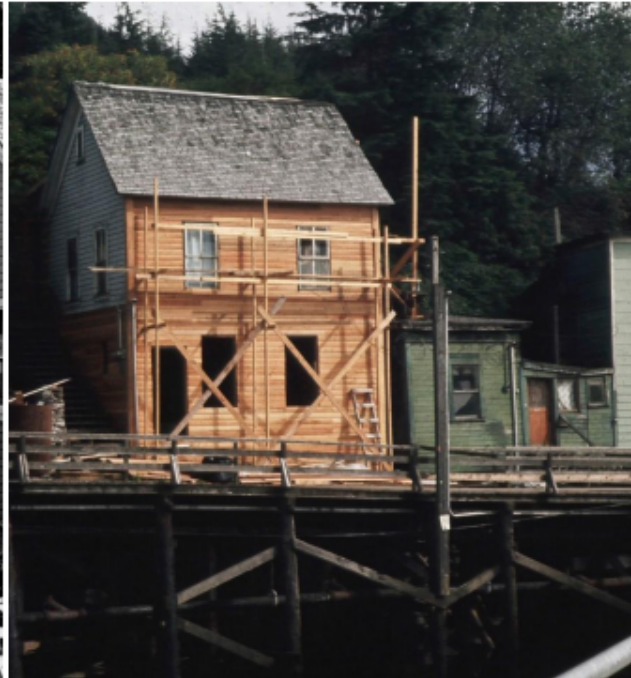
New, locally milled cedar to match original siding was needed to repair deterioration on one facade, 1976. Original windows and trim were also restored.
