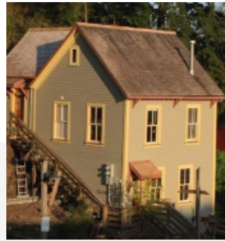
The windows of 28 Creek Street (1902) were replaced in 1976 using all wood replicates and maintaining the original openings and trim. The windows remain in good condition in 2016.
