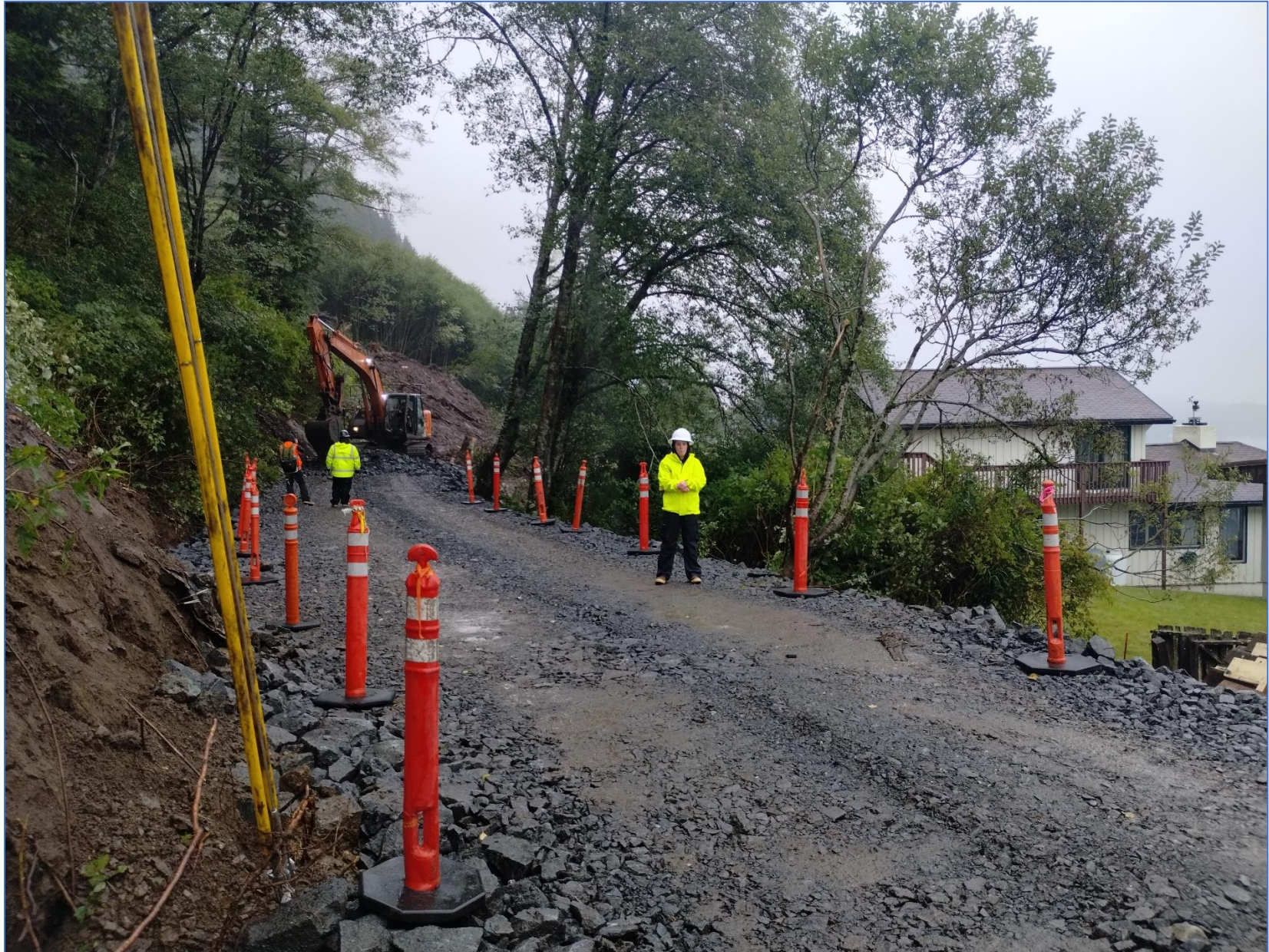
Seccon Construction completing the access road to the debris field. Photo courtesy of ASDF.
