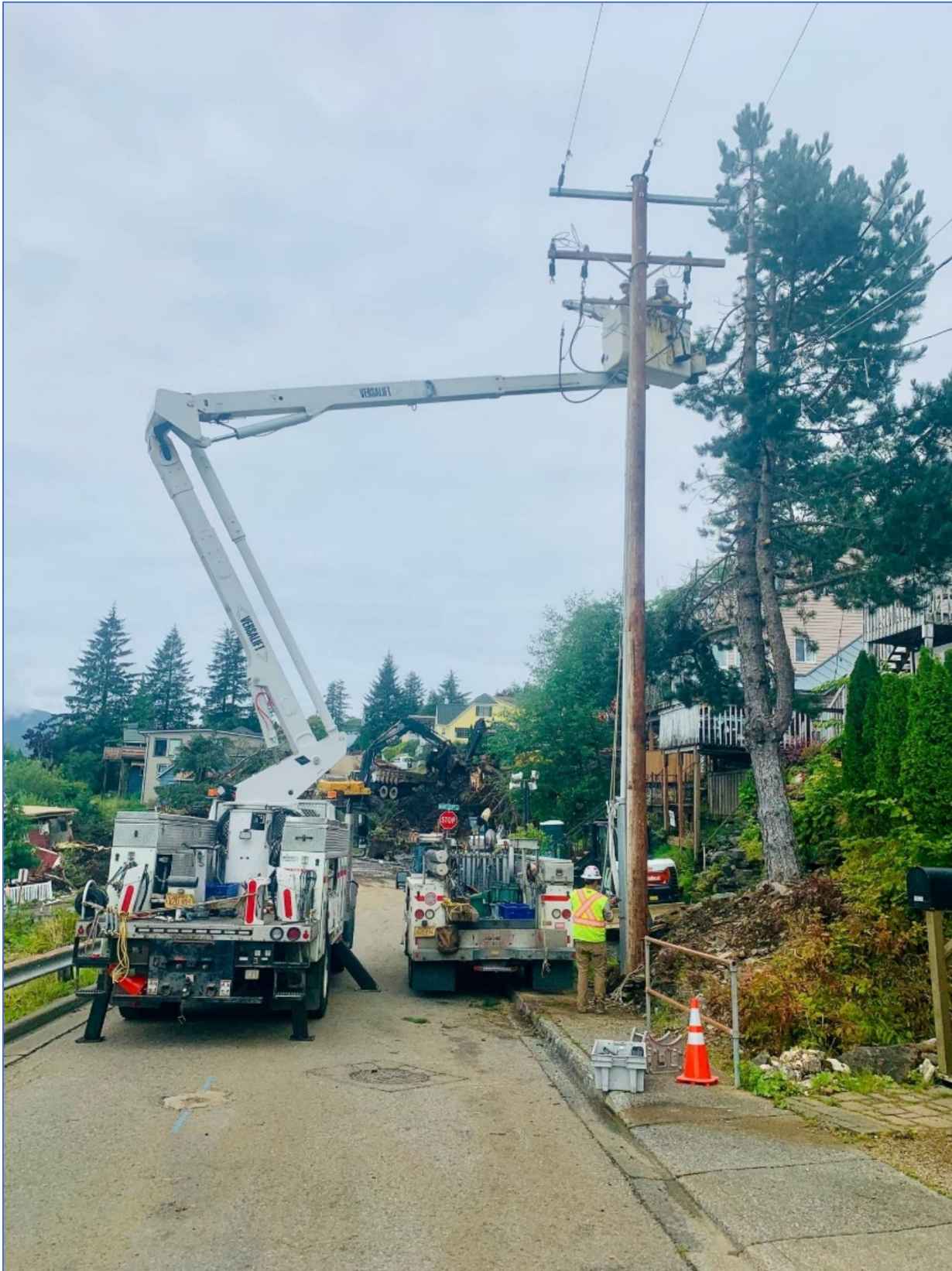
KPU Electric crew replaced a downed electric pole on Second Avenue. Pictured are Nick Kufner, Line Foreman, Donald Munhoven, Service Foreman, and Jerome “Jay” Simmer, Lineman, and Juan “Carlos” Orta, Lineman Apprentice. Photo courtesy of KPU Electric.
