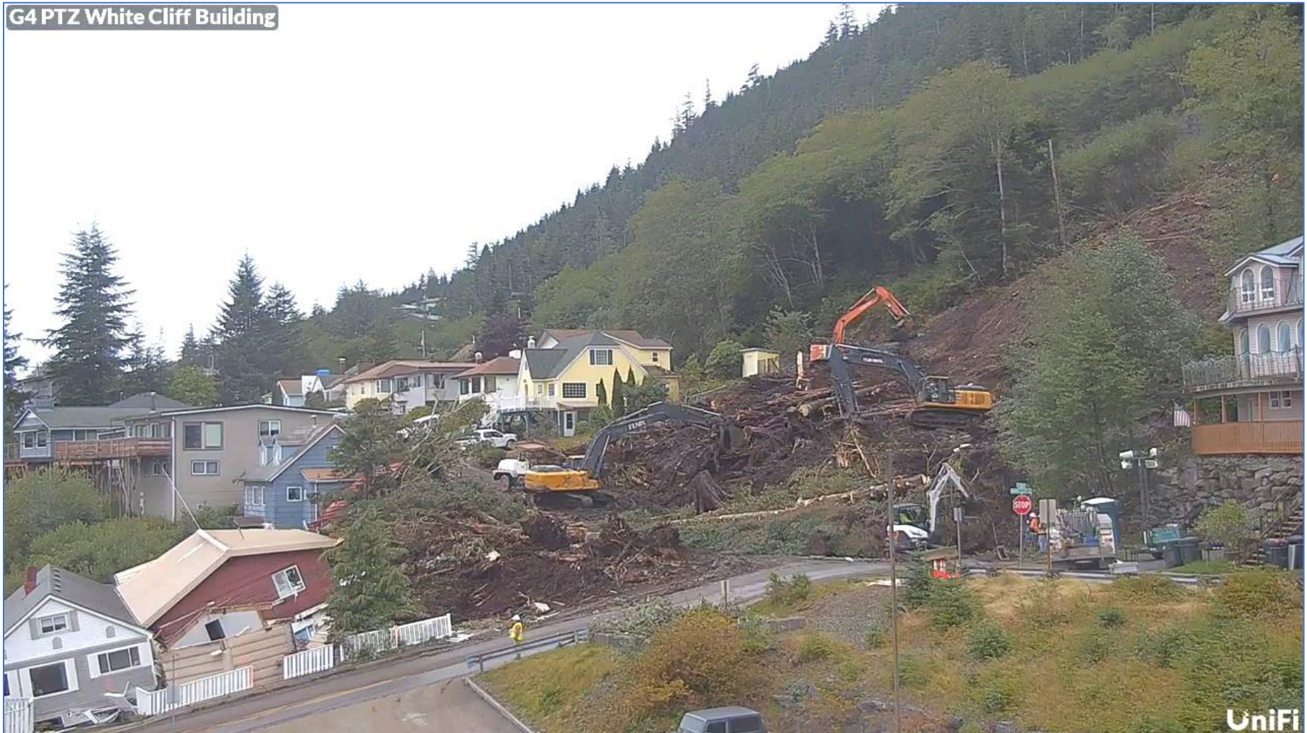
Four excavators and nine dump trucks were on site to remove trees and debris from the Second Ave area. Photo courtesy of the KPU webcam.
