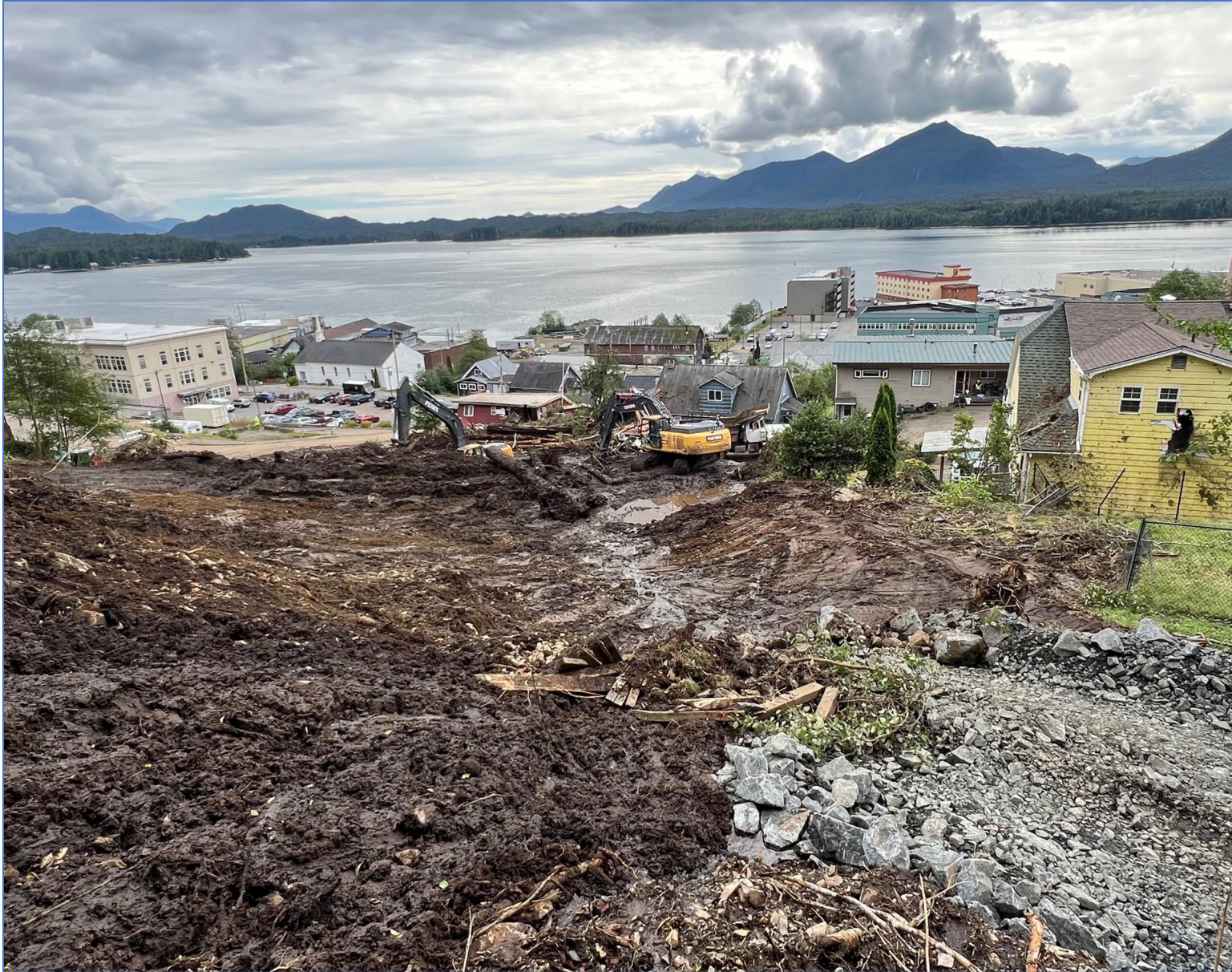
Four contractors and Public Works staff constructed a new access road to clear debris from the slide. Photo credit to City of Ketchikan. Photo credit to City of Ketchikan.
