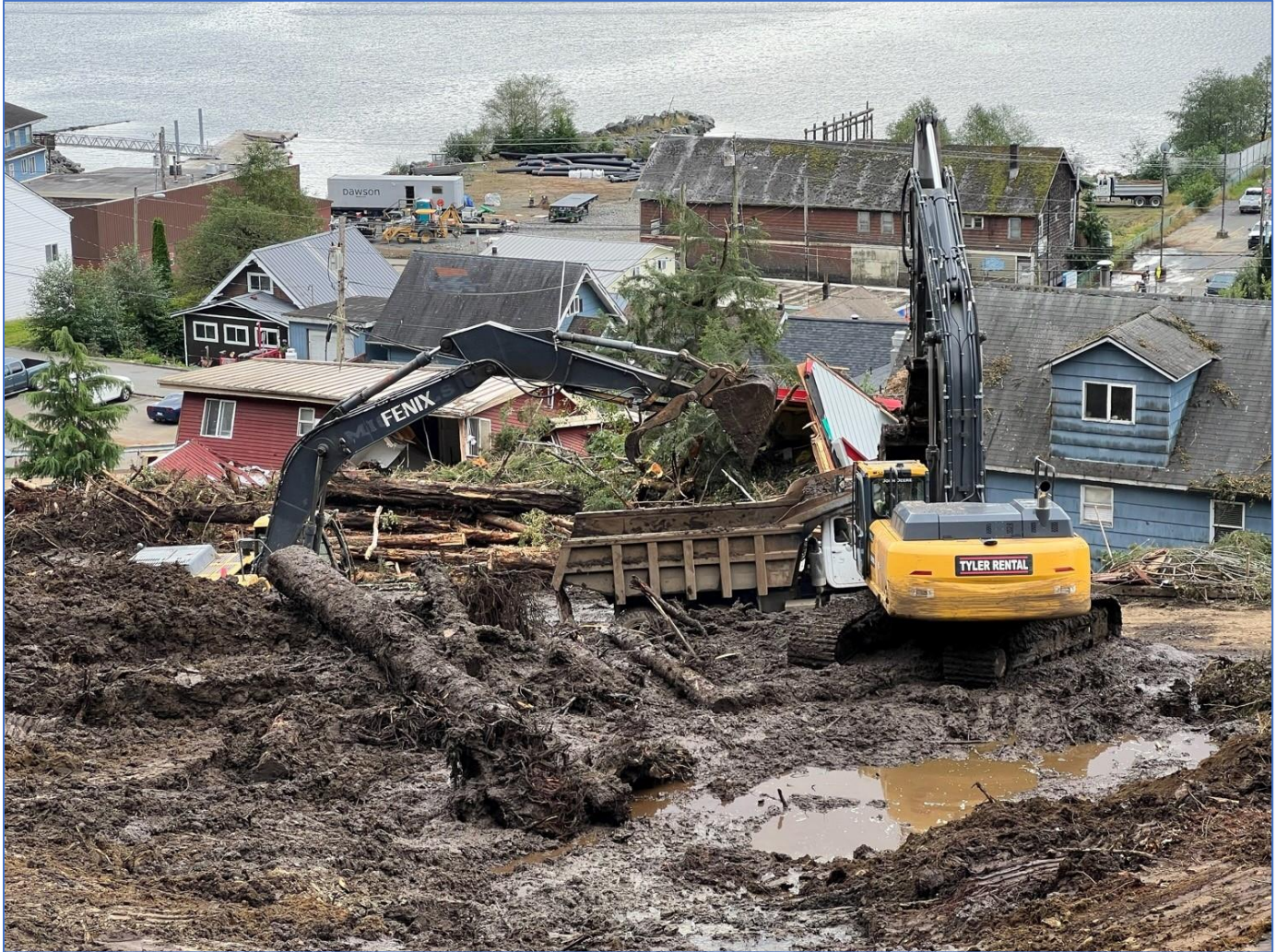
Four excavators and twelve dump trucks were on site to remove trees and debris from the Second Ave area. Photo courtesy of City of Ketchikan.
