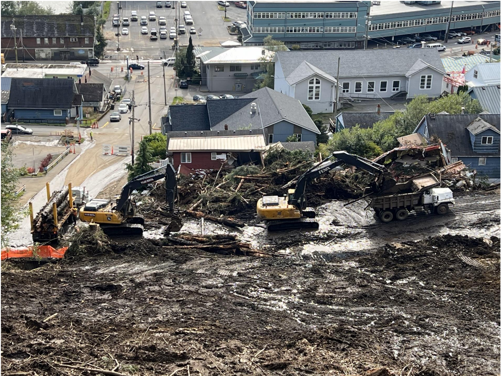
Overview of Second Avenue with contractors clearing trees and debris. Photo courtesy of City of Ketchikan.
