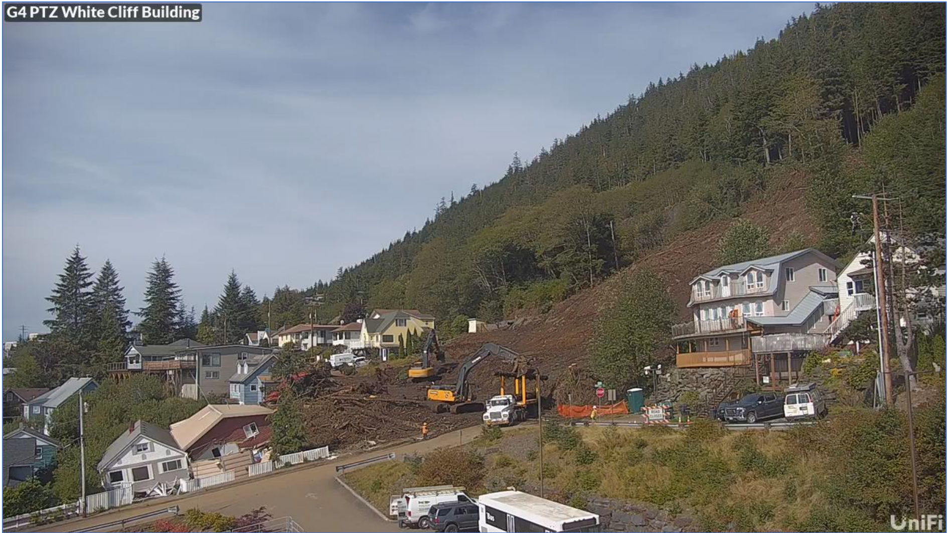
Contractors removing downed trees from the debris field on Second Avenue. Photo courtesy of City of Ketchikan.
