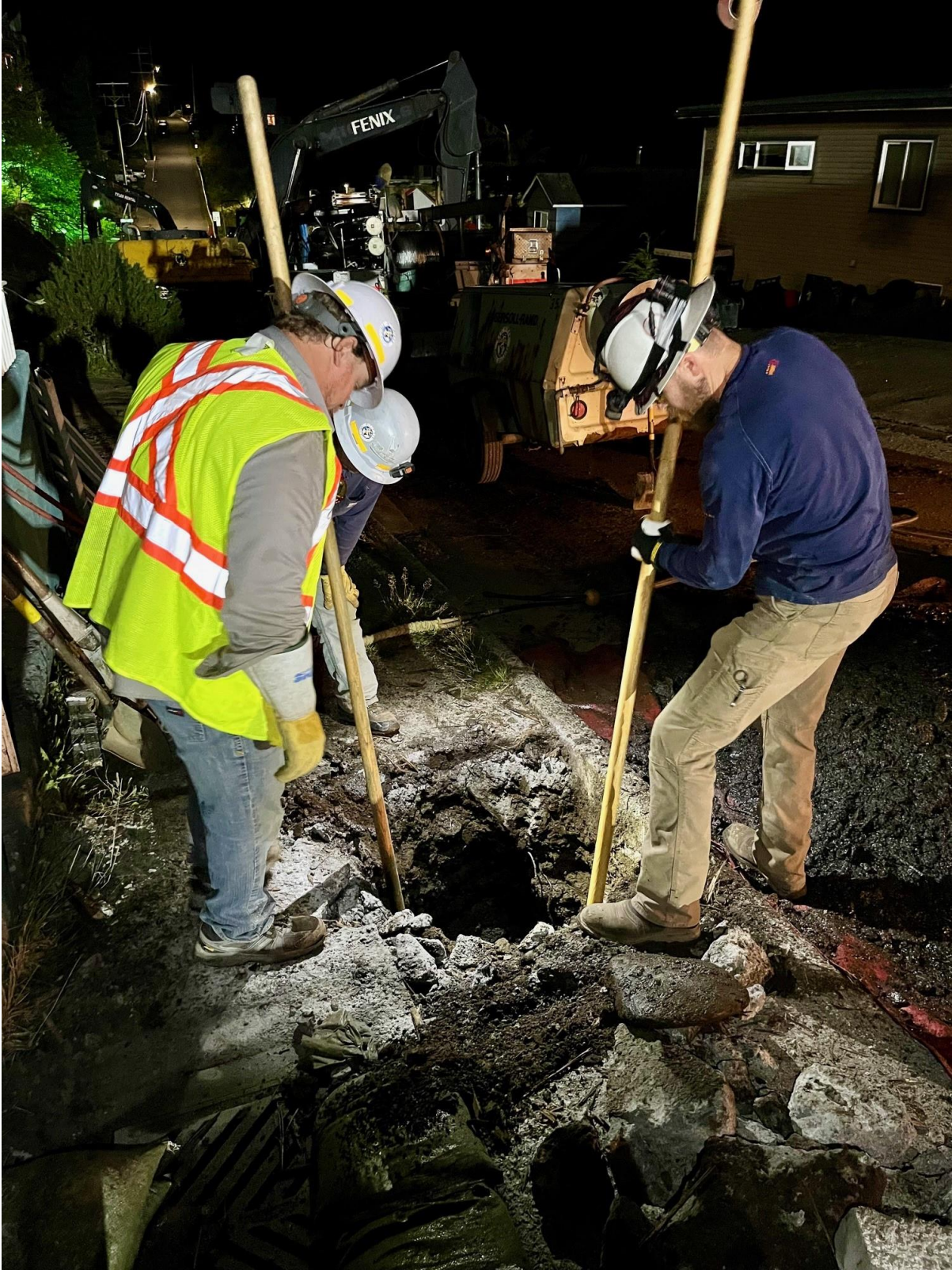
KPU Electric crew working to clear the damaged electric pole. Photo courtesy of KPU.
