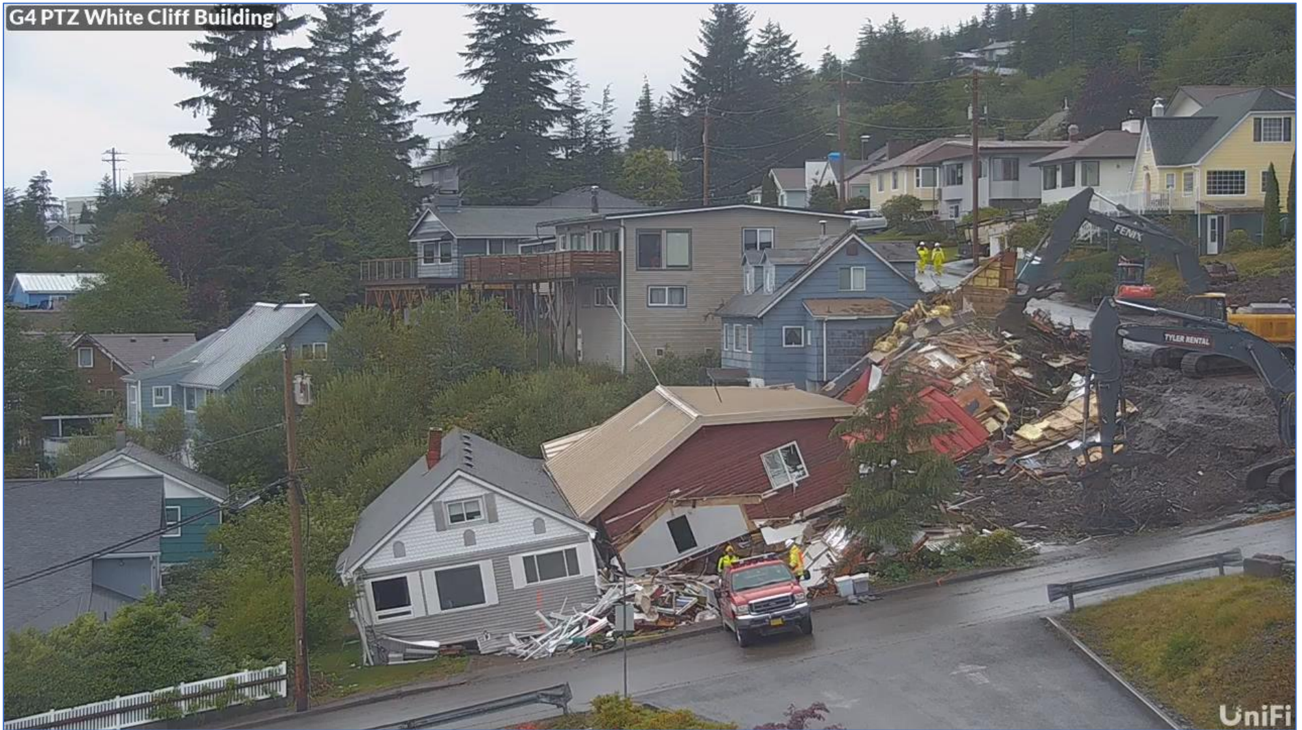
Safety Officers observing operations on Second Avenue and White Cliff Avenue. Excavators removing house debris from the top of White Cliff and Second Avenues, and Fire Department crew removing household items from the second collapsed home.
