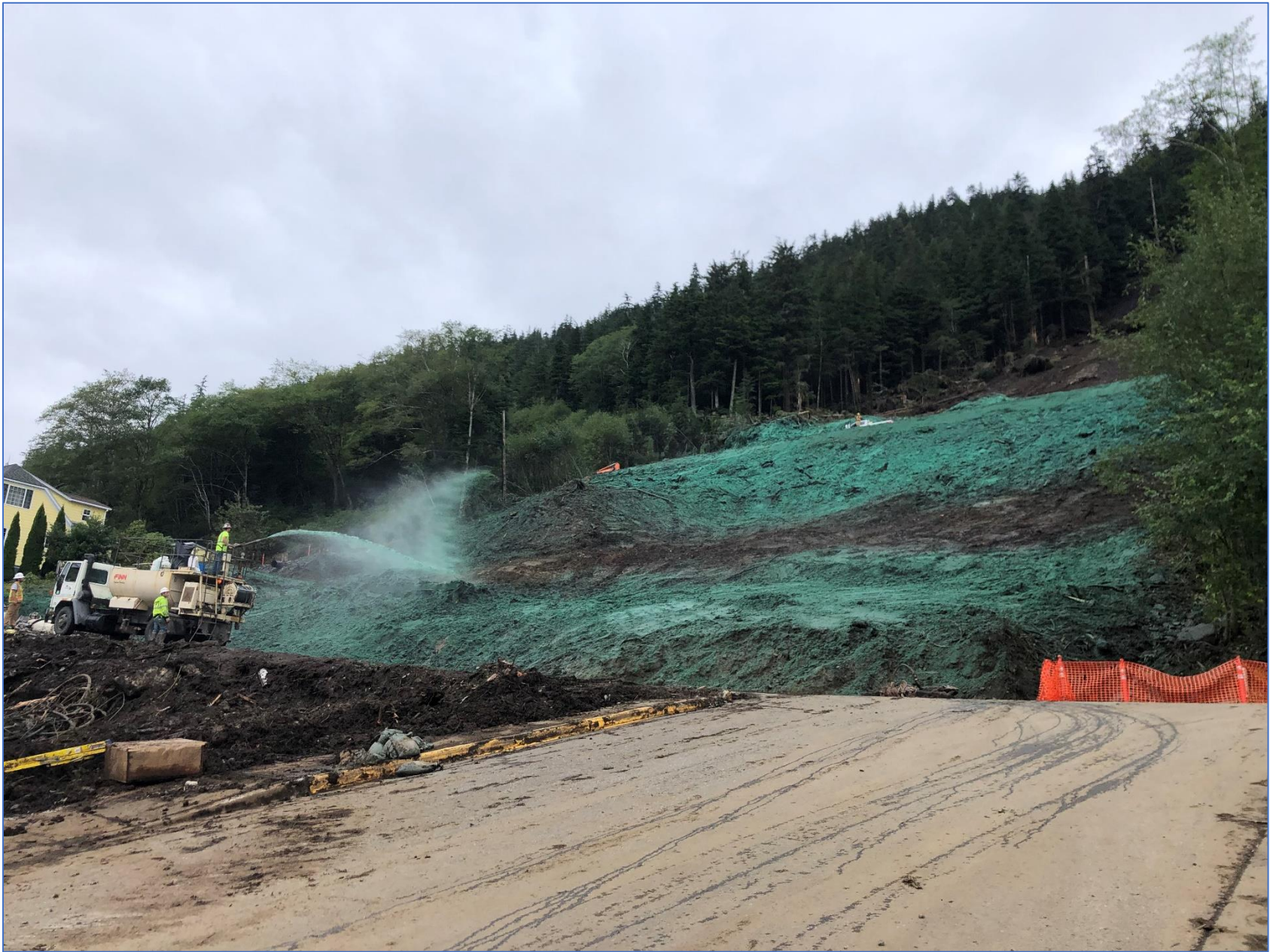
Seccon Construction crew applying hydroseed to the slope above Second Avenue. Photo courtesy of KGB.
