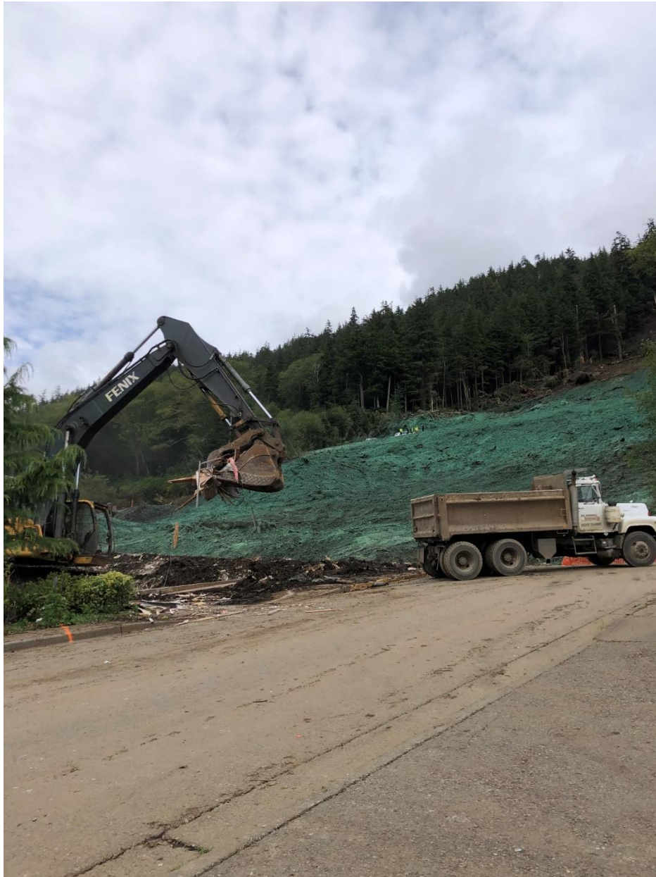
Robert McRoberts loads house debris into a dump truck on Second Avenue. Photo courtesy of KGB.
