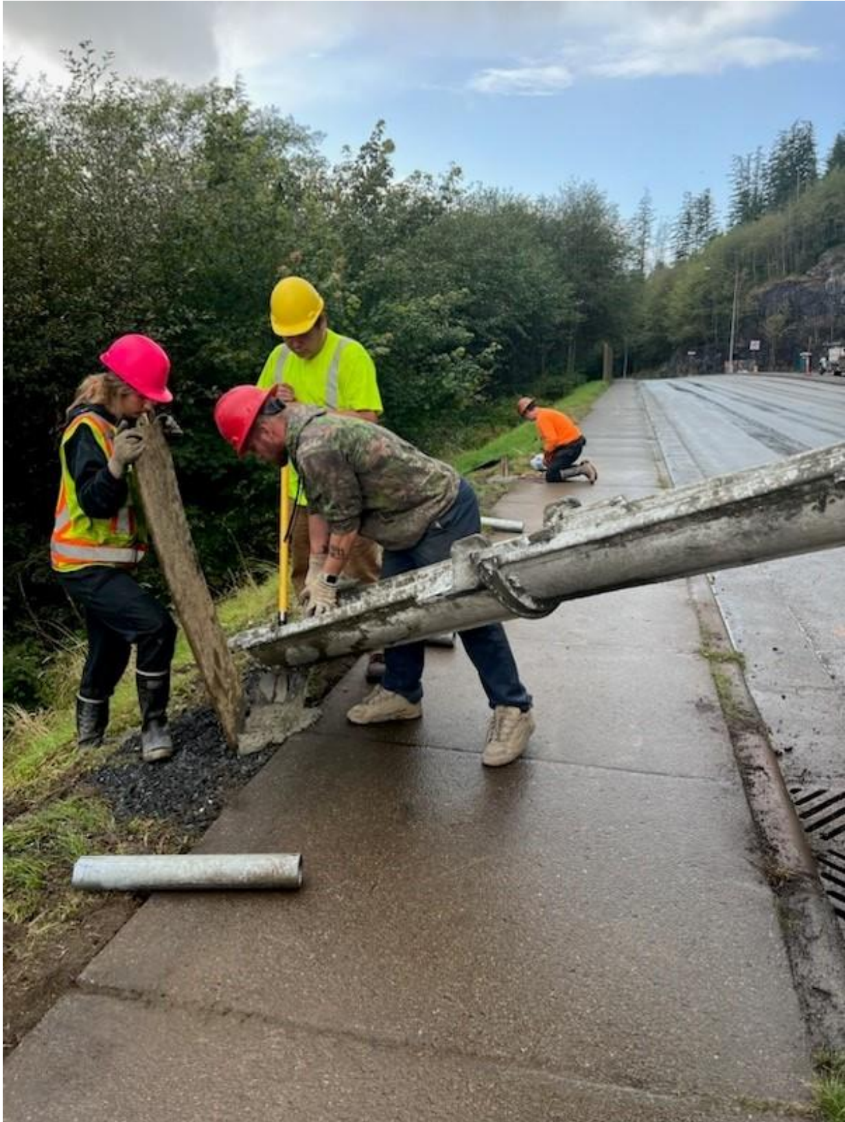
Work crew pouring concrete into fence post base on Third Avenue Bypass. Photo courtesy of City of Ketchikan.
