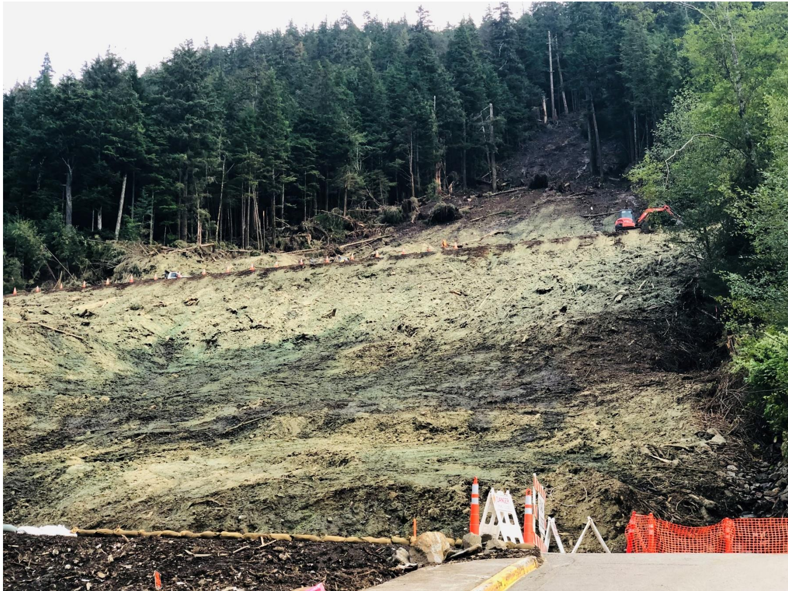
View of Third Avenue Bypass from White Cliff Avenue. Crews work to install fence post bases. Photo courtesy of KGB.
