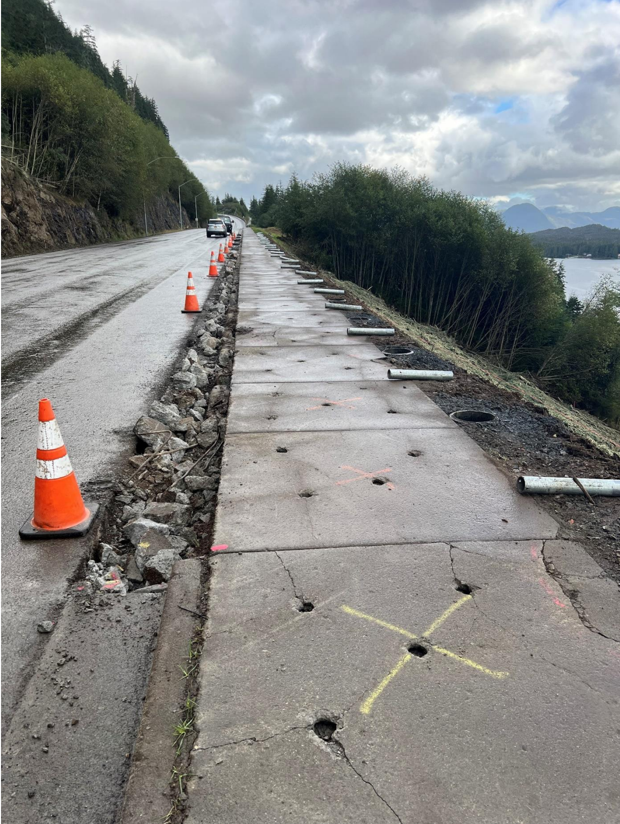
Fence post bases are installed on the Third Avenue Bypass. Photo courtesy of City of Ketchikan.
