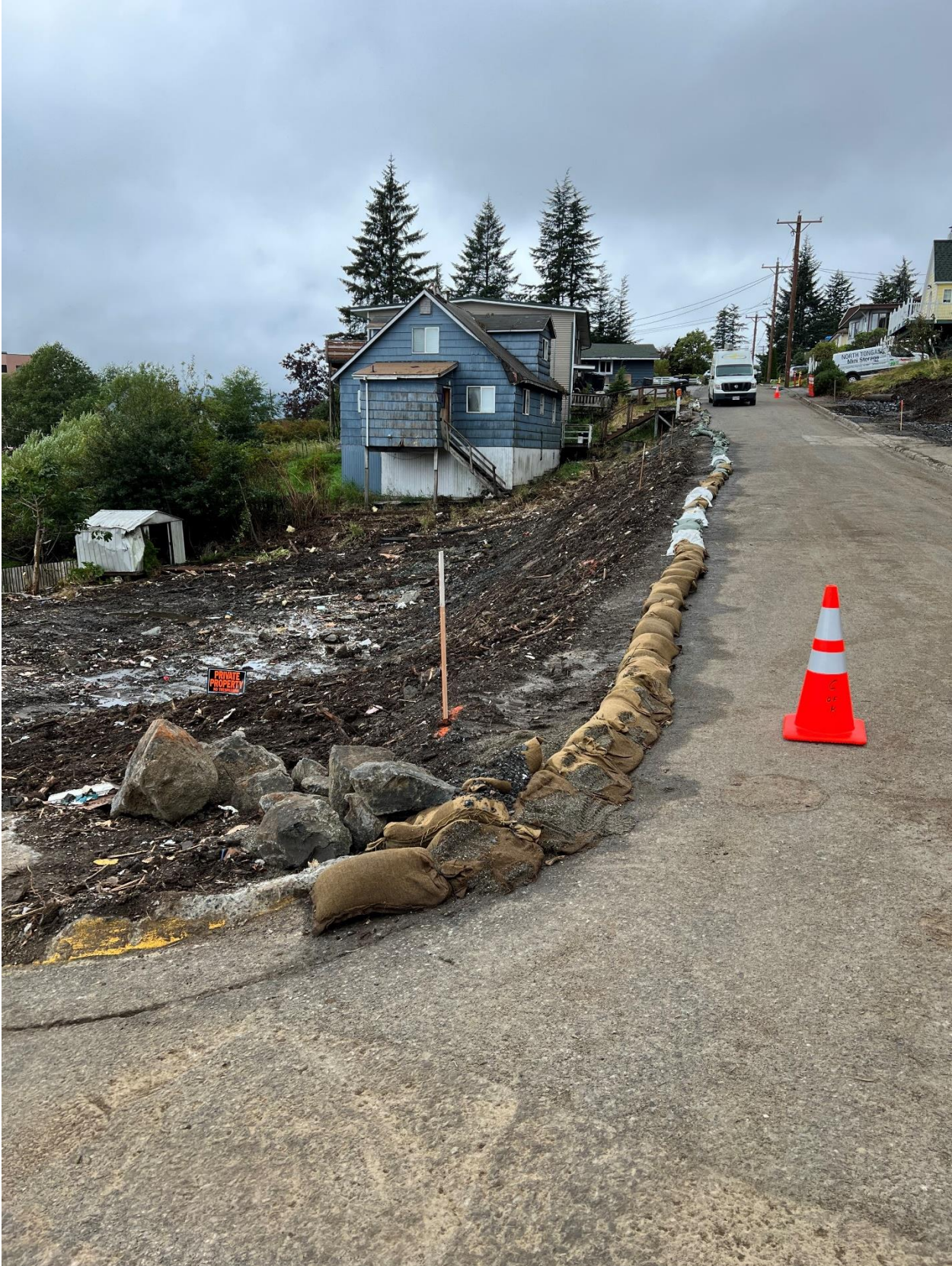
Sandbags placed to control storm water on Second Avenue. Photo courtesy of City of Ketchikan.
