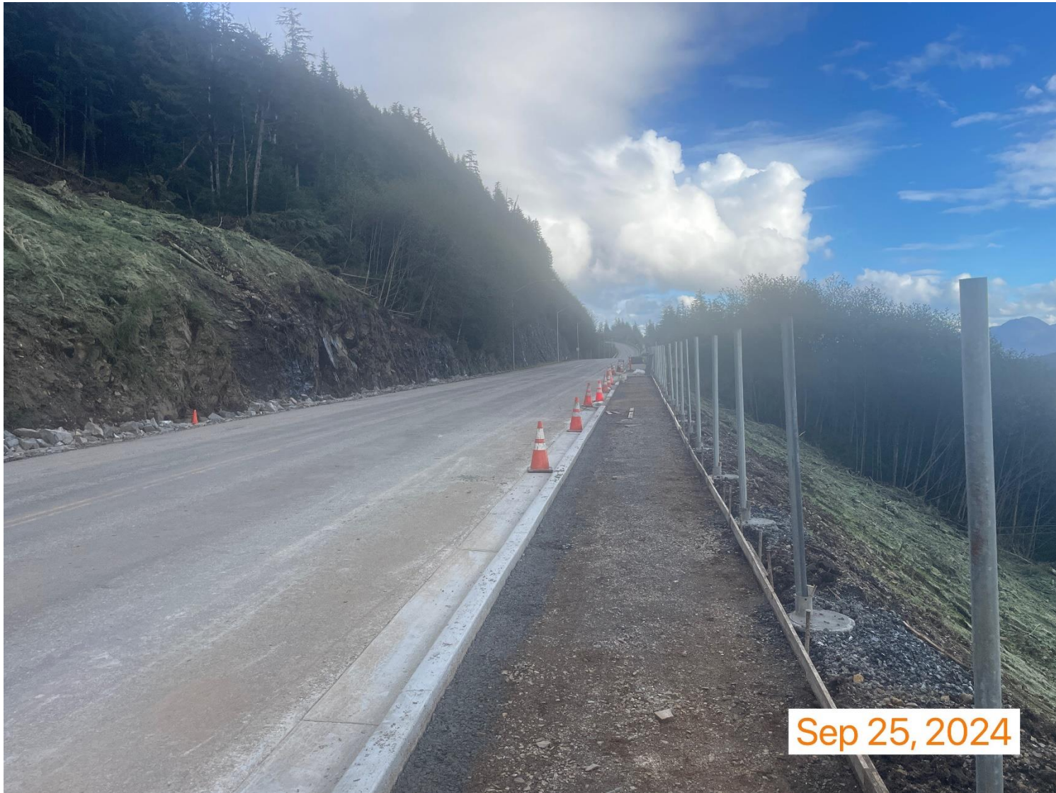
New fence posts installed, and preparations for new sidewalk to be poured. Photo courtesy of City of Ketchikan.
