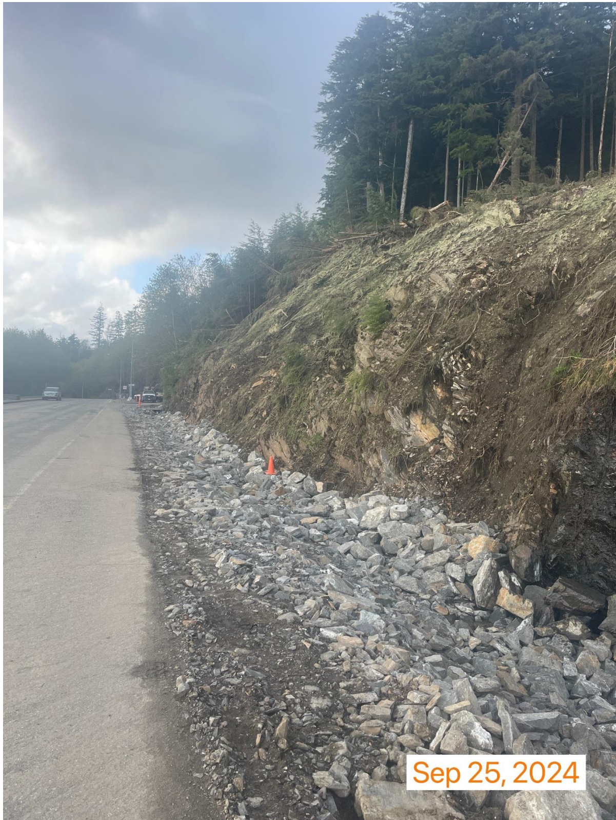
Rock added to the base of the slope above the Third Avenue Bypass. Photo courtesy of City of Ketchikan.
